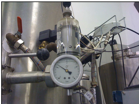
Figure 3: Position of SENSOR2 on the carbon dioxide outlet valve assembly. The sensor can be seen below the gauge dial, glued upside-down to the bottom of the assembly. Photo by D. Varner
